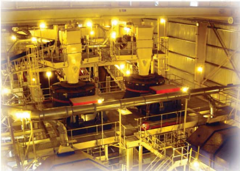
Two Turbo™ 160's installed in a Power Plant Crushing Gob Coal For Fluidized Bed Combustion. This Power Plant Burns 1000 TPH 24 Hours a Day / 7 Days a Week.
